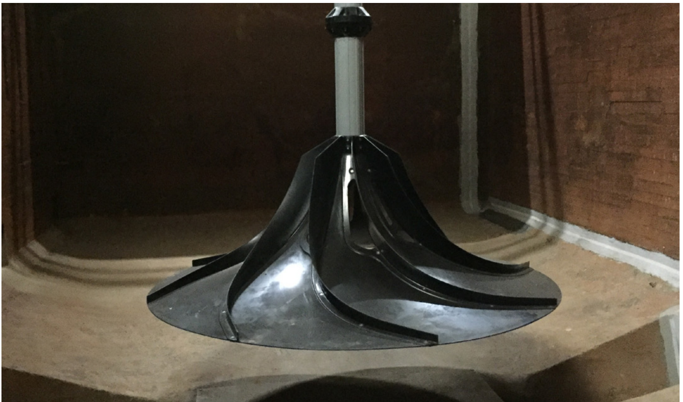
INVENT HYPERCLASSIC® mixers in the flocculation tank in the Vanhakaupunki drinking water treatment plant, Helsinki, Finland
