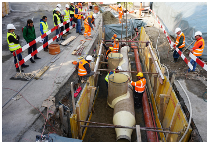
Figure 2: A new GRP Combined Sewer Overflow chamber separates suspended solids from the wastewater network in Castel San Pietro (Switzerland)
