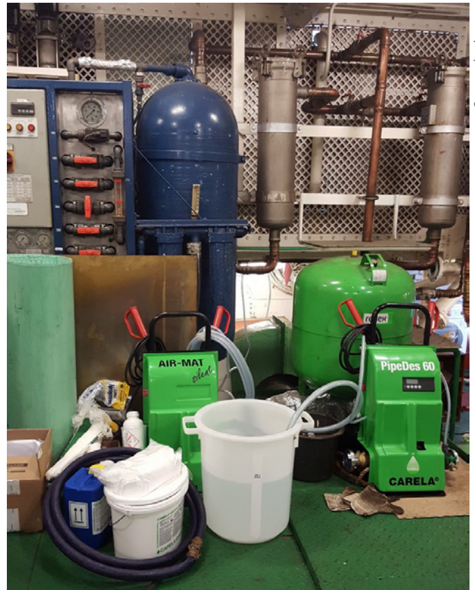
Equipment for cleaning on board
