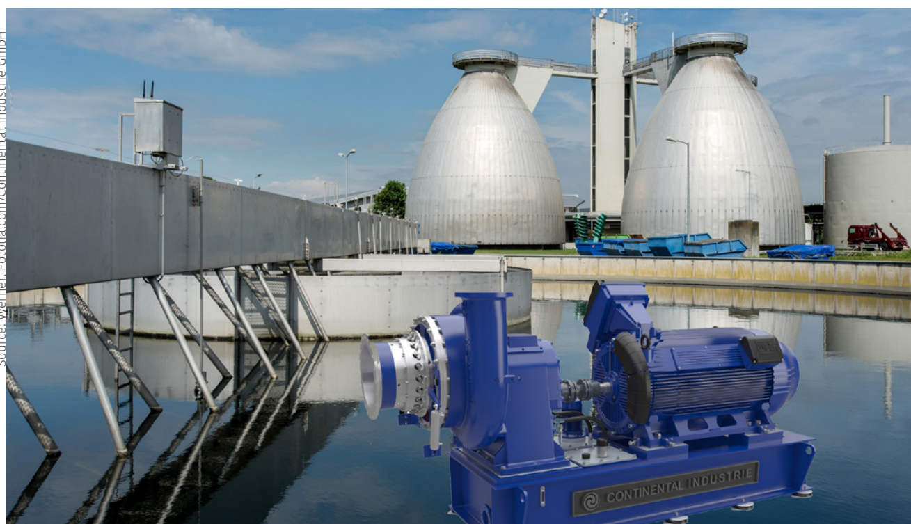
Wastewater treatment plant
