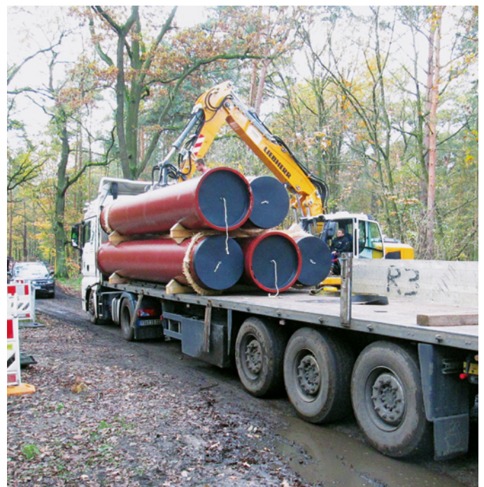
Figure 7: The 6 m long pipes are delivered direct to the construction site by truck
