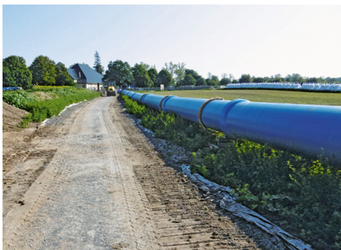
Figure 2: The route of the DN 800 interim pipeline over the dike between the pipe bridge over the River Mulde and the Canitz waterworks
