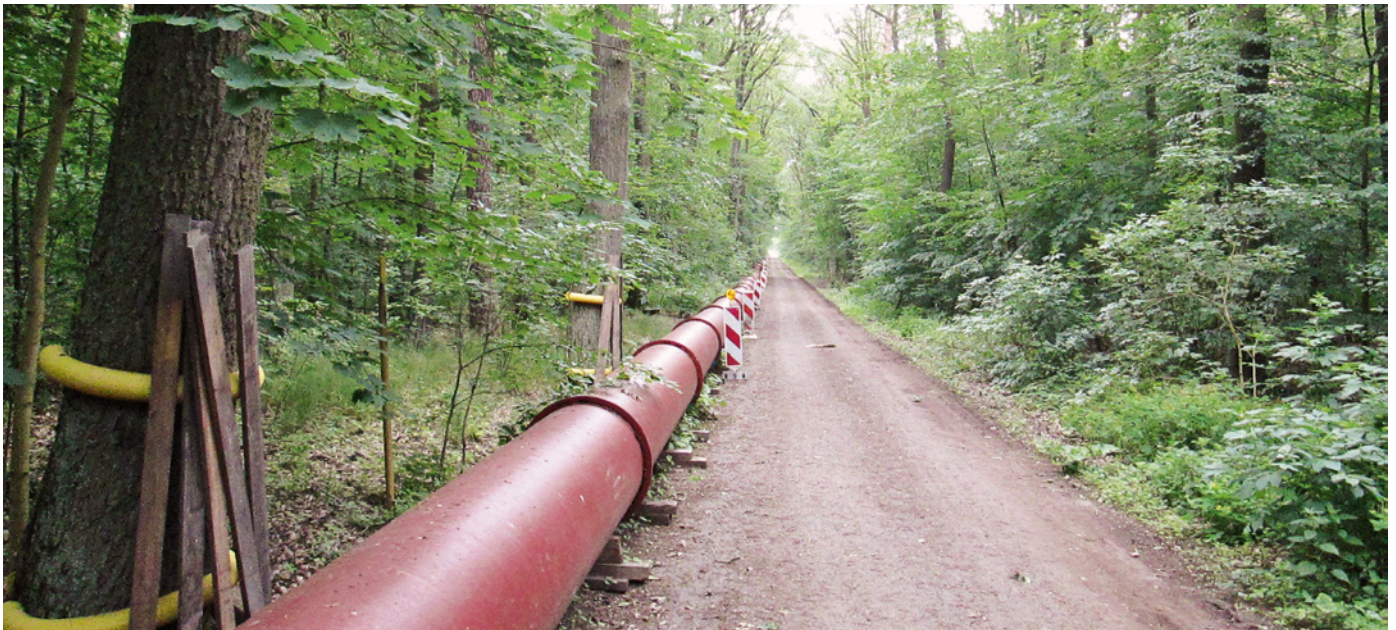
Figure 6: Environmentally friendly and space saving construction of the interim pipeline along a forest road
