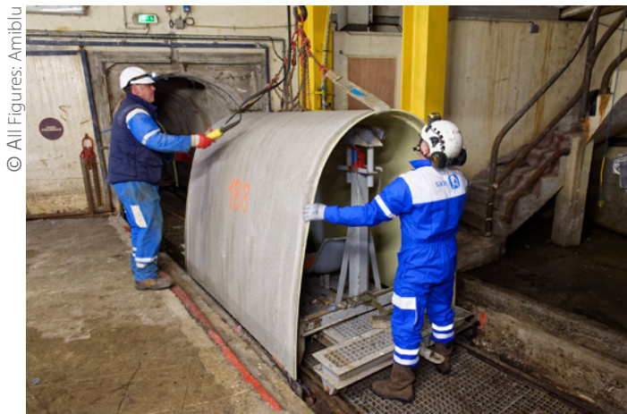
Figure 1: In the surroundings of Toulon (France), 2714 GRP half-shells were installed to rehabilitate an aged sewer system
