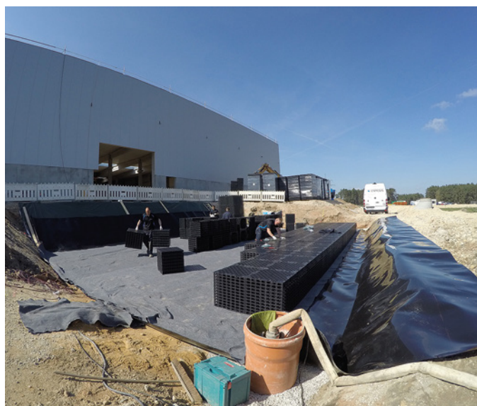
ENREGIS' installation team implementing the retention system on the site in Röttenbach, Germany
