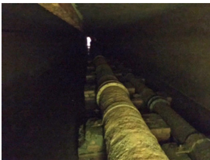
Figure 1: One hundred year old 18 inch water pipe running directly under the runway of major airport
