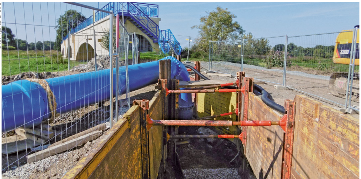
Figure 1: Excavation pit with a DN 800 interim pipeline coming out of it and onto a pipe bridge over the River Mulde
