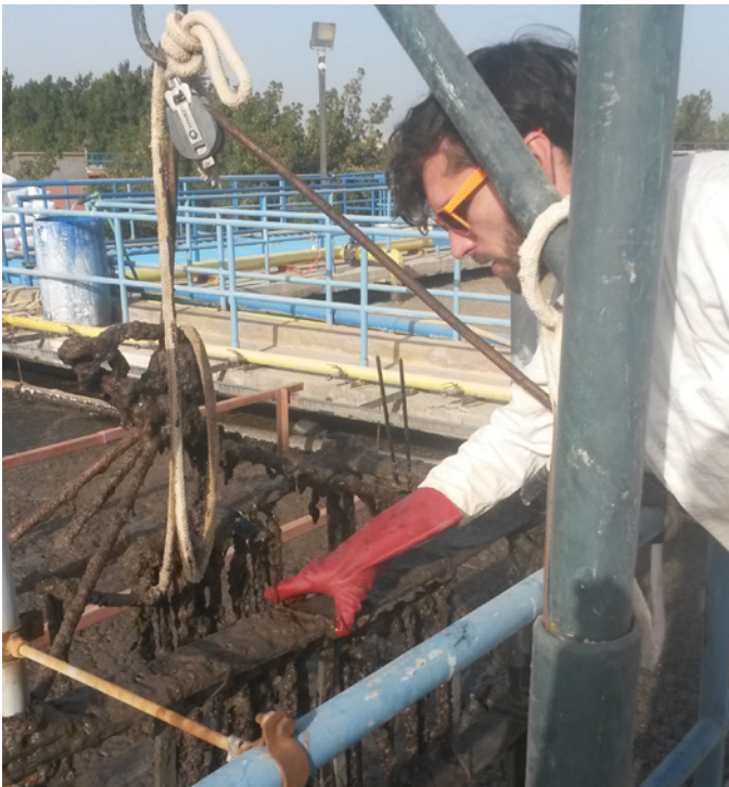
Figure 4: Implementation of biofilm carrier material in the wastewater treatment plant
