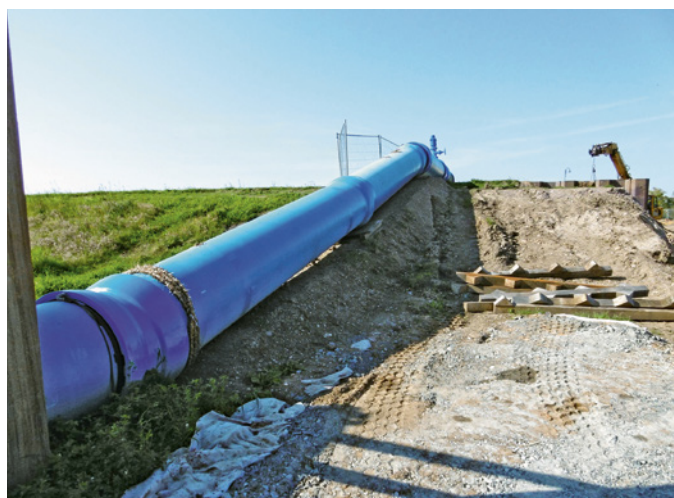
Figure 3: The straight section of the interim pipeline along the construction road to the Canitz waterworks
