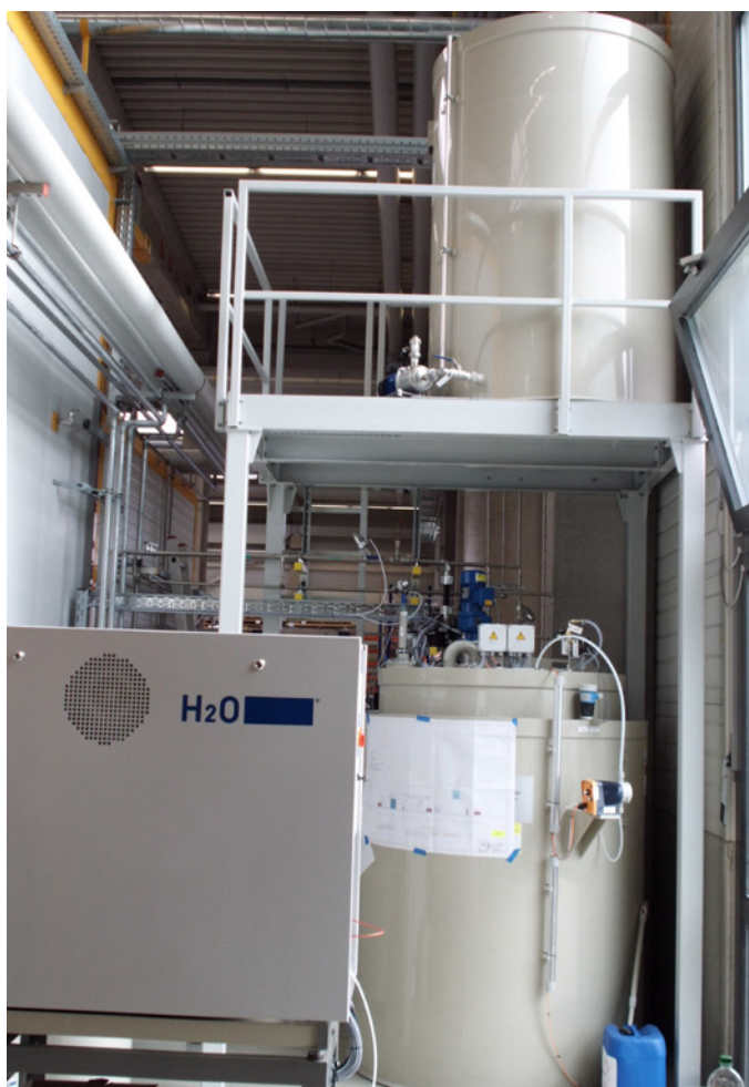
Tight spaces are not a problem for H2O GmbH's engineers: The tanks were quickly placed on top of one another to save space in the production facility
