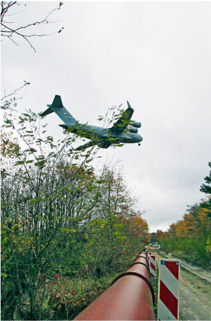
Figure 4: Interim pipeline along the route of the sewage pressure pipeline to be renovated in the approach path to Berlin Tegel Airport
